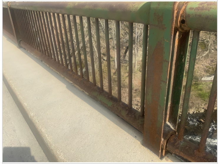
Section loss upstream rail
