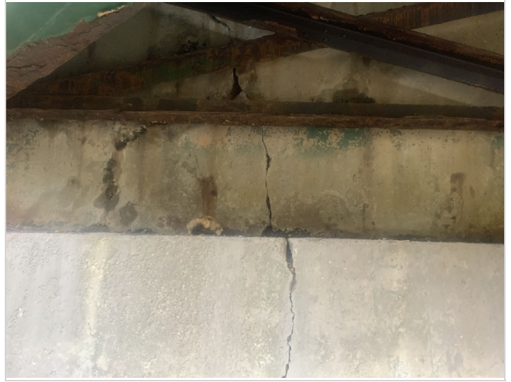
Vertical crack abutment 2
