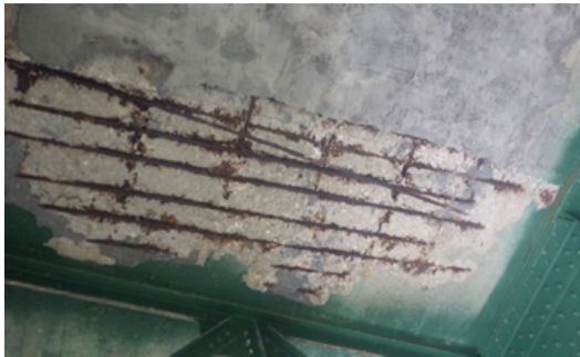
Fig. 4 - Typical Exposed Deck Reinforcing Under Deck
