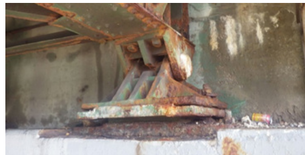
Fig. 3 – Typical Deterioration of Bridge Seats, Bearings, and Beam Ends
