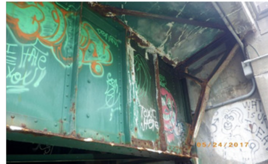
Fig. 5 - Typical Deterioration of Sidewalk Supports
