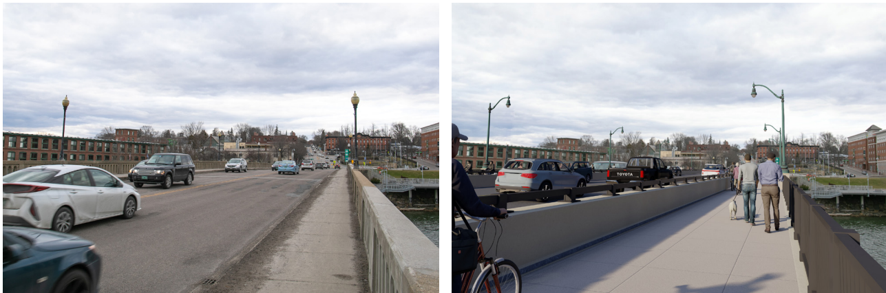
Fig. 17 - Existing and Proposed Bridge Sections - The Shared Multi-use Path Increases Pedestrian, Bicycle and Vehicle Safety
