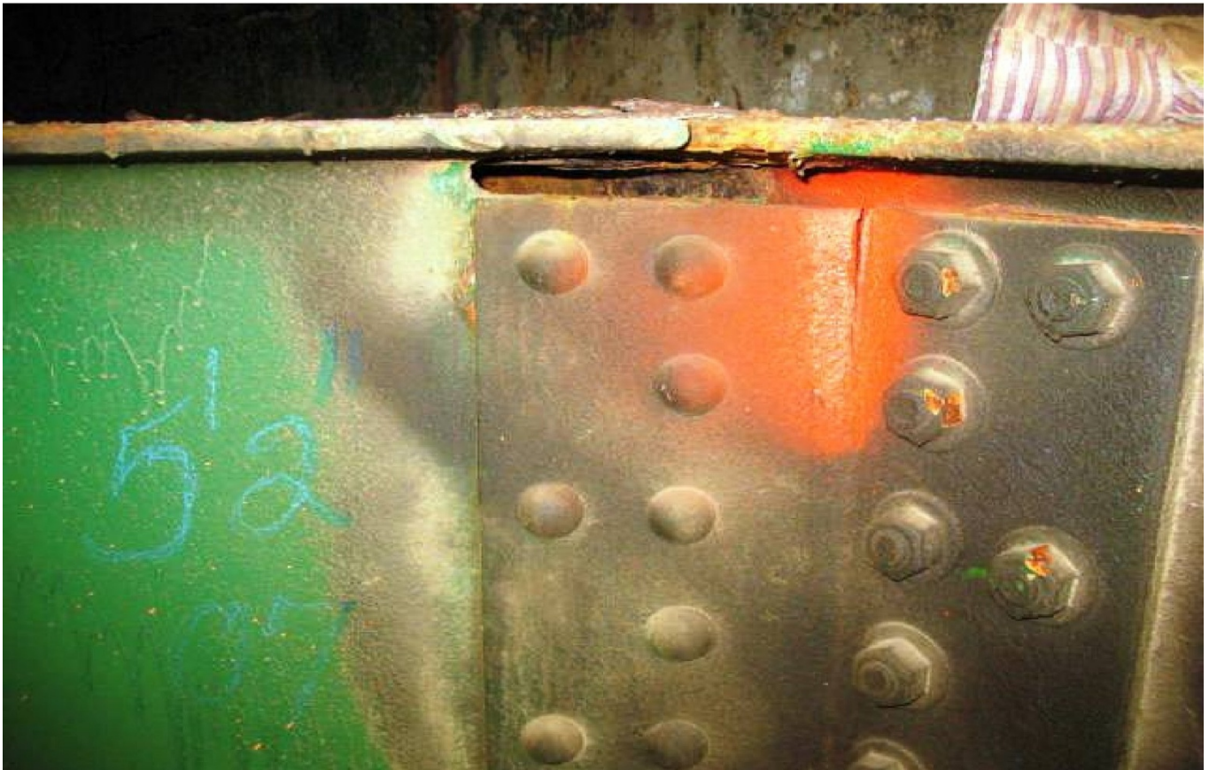
Secondary Member Crack
