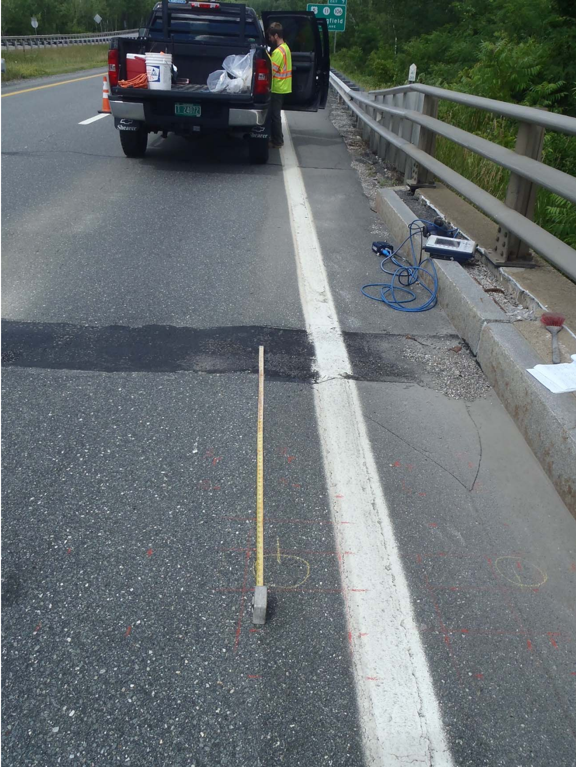
File picture showing the GPR unit used and typical grid pattern determined from GPR to avoid coring rebar.
