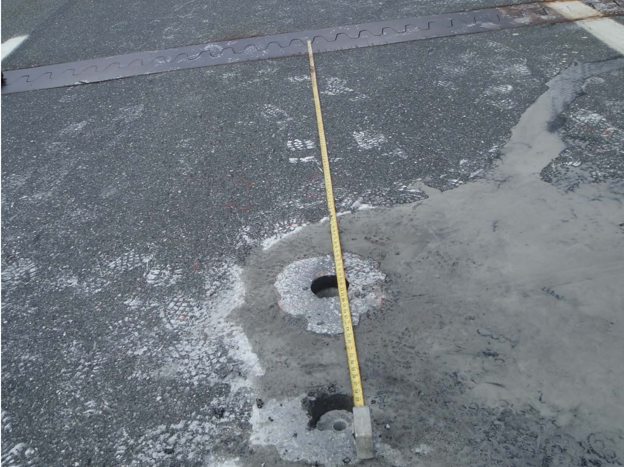
Sample area 2 core location 3, approximately 8 feet south of hinge joint on second span
