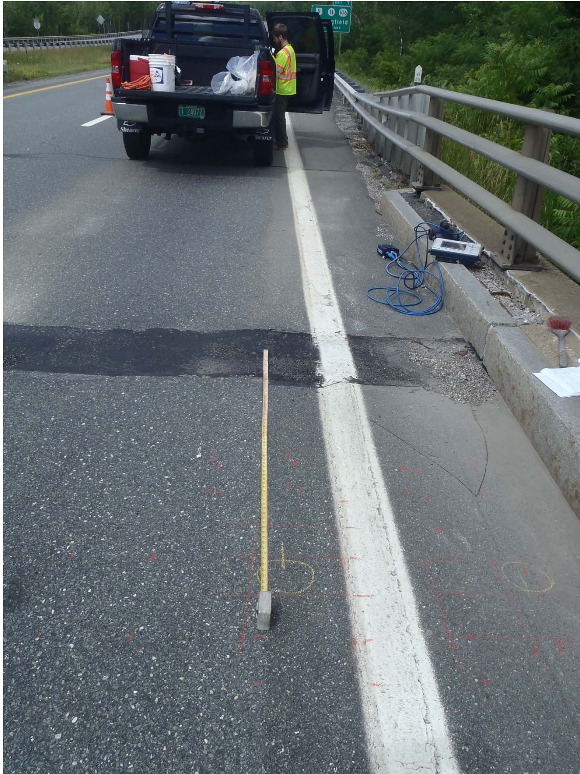
Sample area 1, North end of the bridge. GPR unit, on the curb, that was used to layout the rebar grid prior to coring
