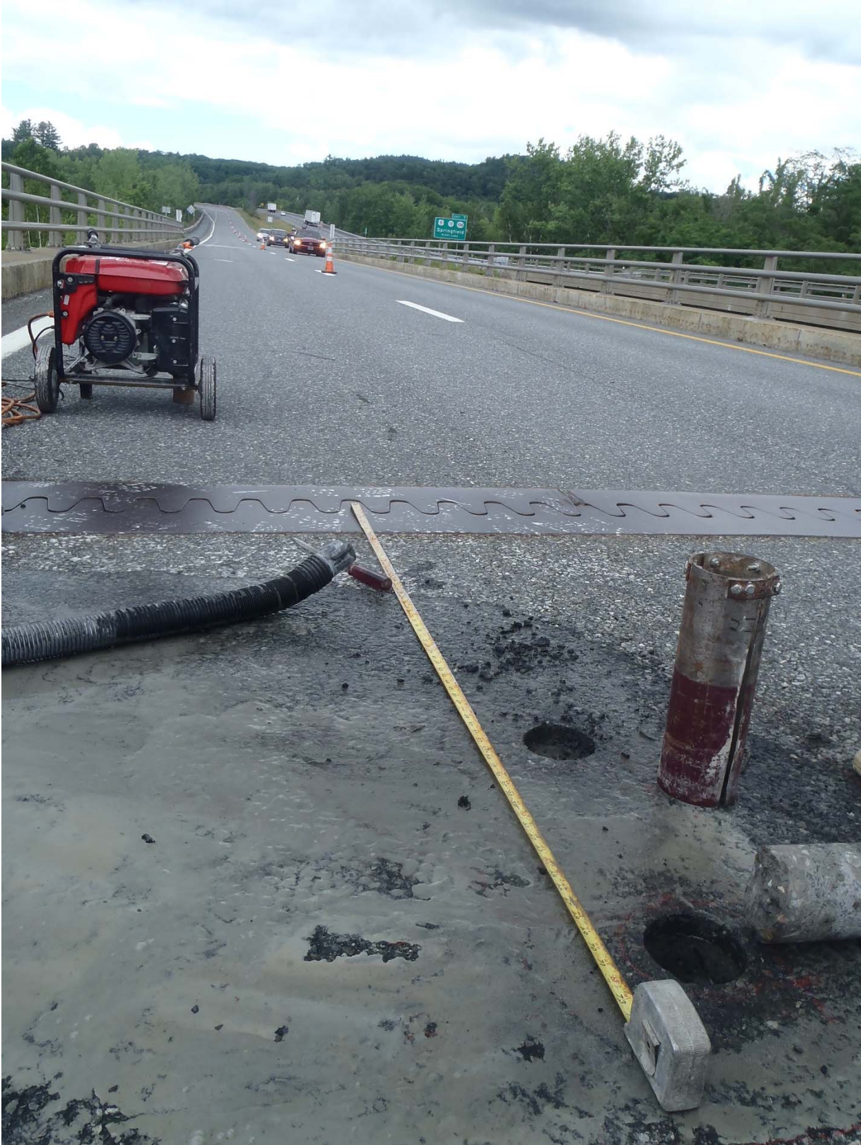
Sample area 2 core location 3, approximately 8 feet south of hinge joint on second span
