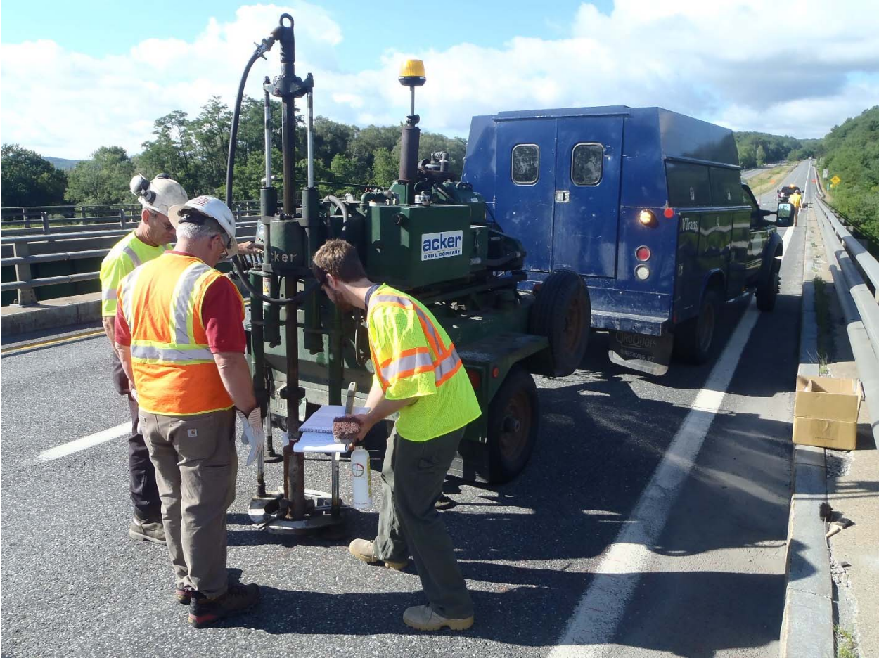
Trailer mounted core rig used by Vtrans Drilling unit used to cut the cores.
