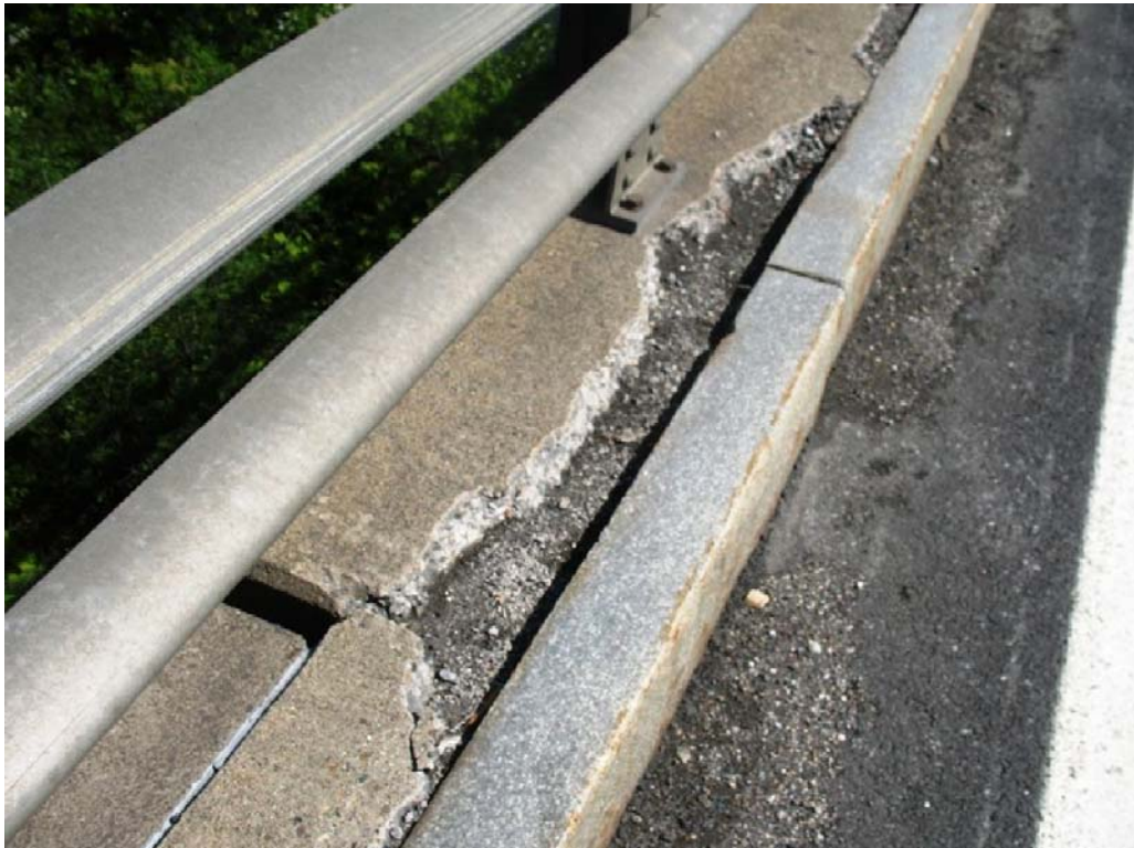
Bridge Curb Deterioration (Bridge 26S shown)
