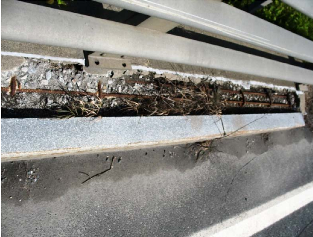
Bridge Curb Deterioration (Bridge 26S shown)
