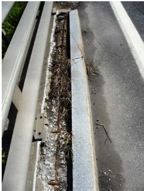
Figure 2: BR 26 S Curbing Requiring Patchwork
