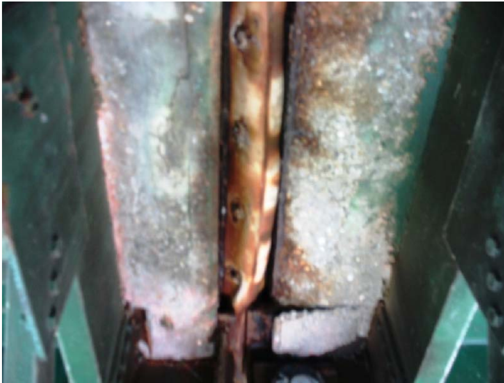
Deck Condition at Expansion Finger Joint, Located above Hinges (Bridge 26S shown)
