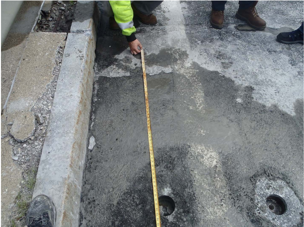
Sample area 1, North end of the bridge. measuring from end of bridge to core hole locations
