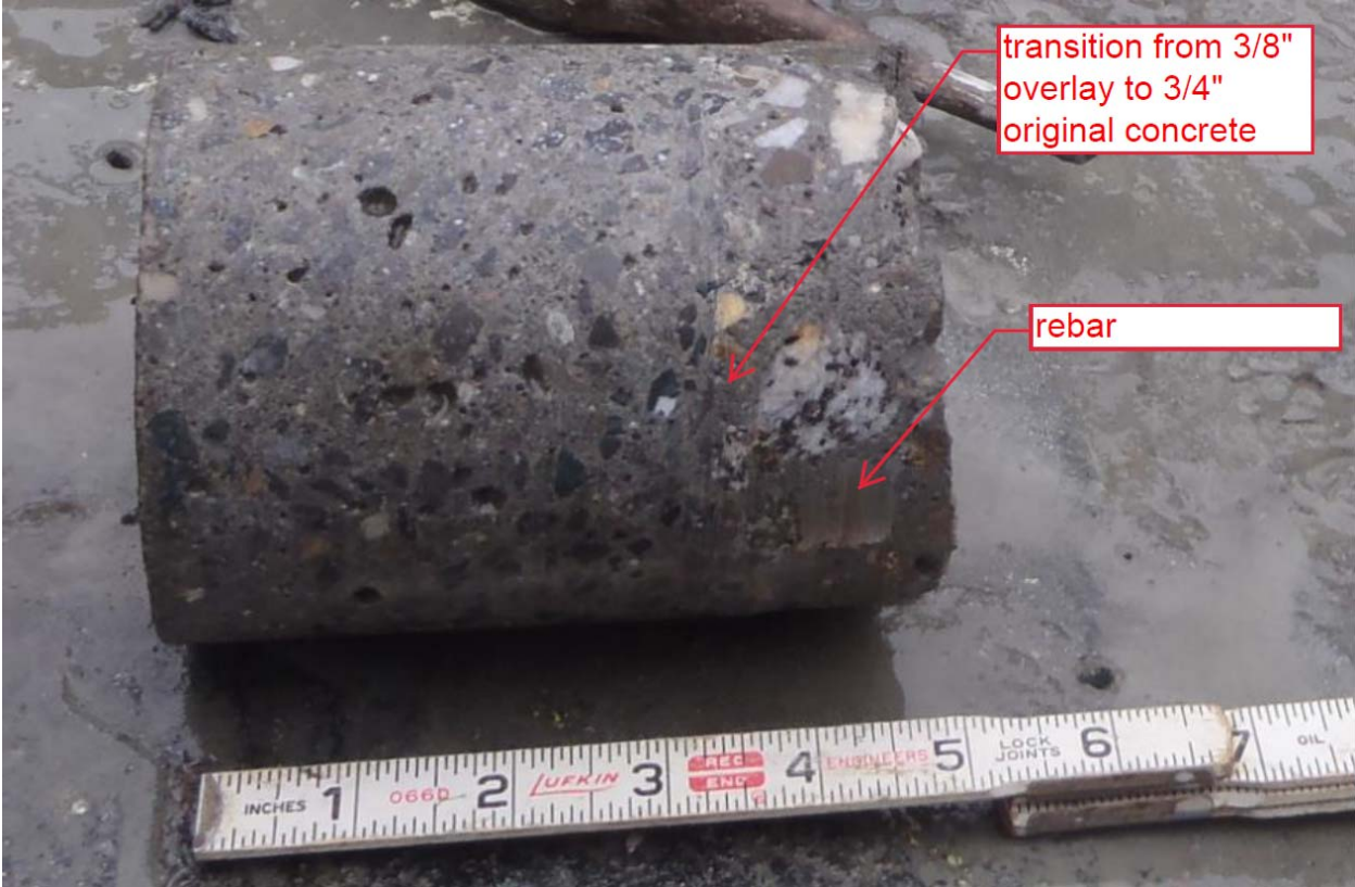
Core 1B showing interface of 3/8" aggregate concrete to 3/4" concrete.
