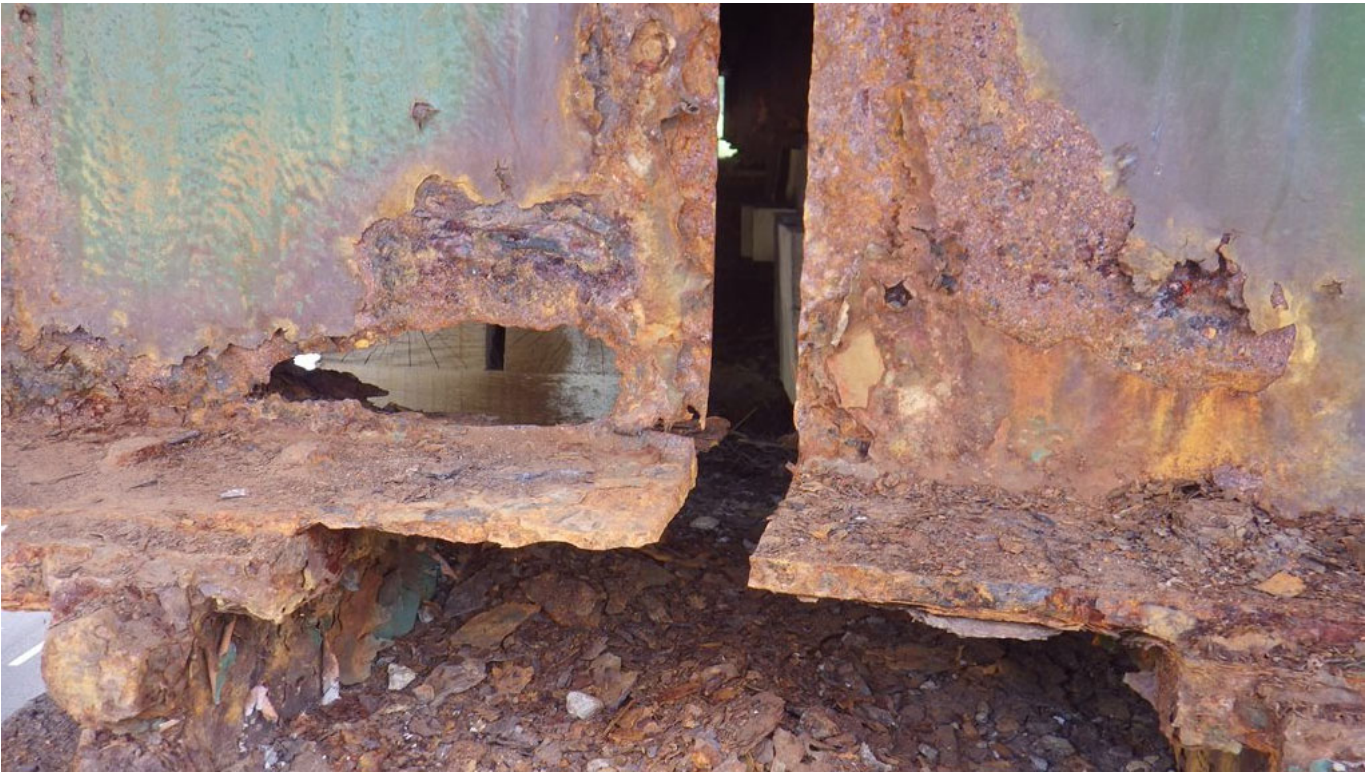
Rolled beam deterioration at joint
