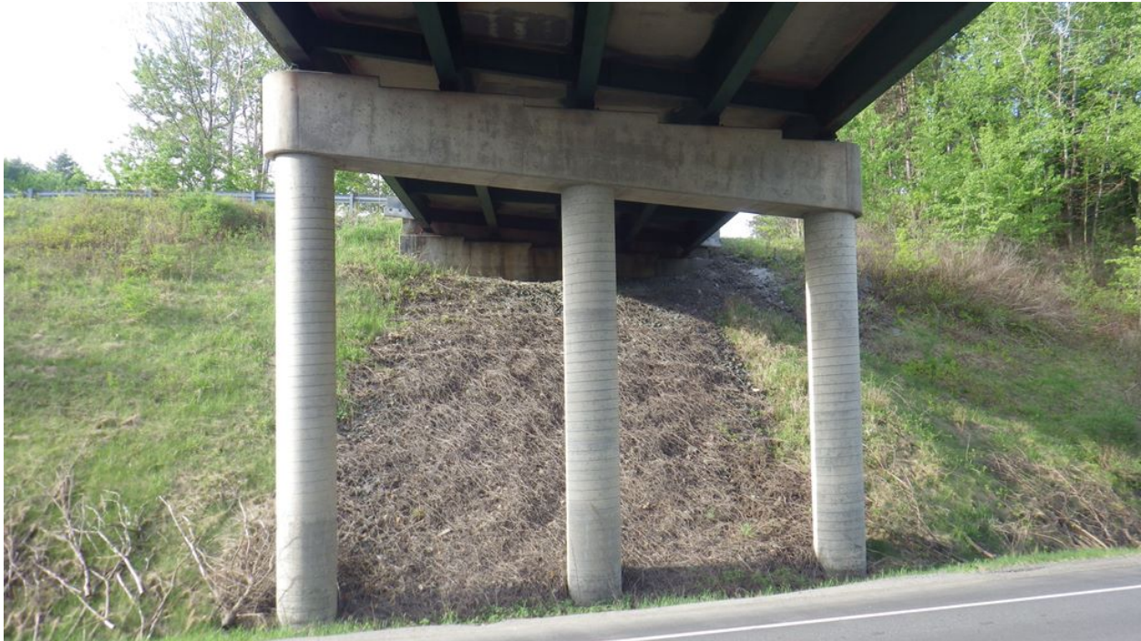
Figure 3.1: Stone fill armoring at bridge abutment underneath Interstate 91 Bridge 28 Southbound. [Inspection photo dated 2018]
