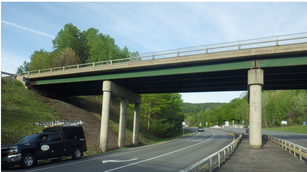
Figure 3.2: Facing I-91 Bridge 28 Southbound south abutment; note limited overhead clearance for drilling operations under existing bridge. [Inspection photo dated 2018]
