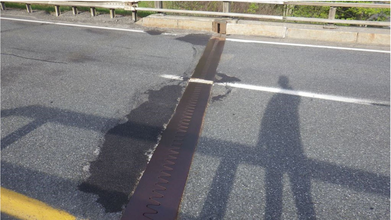
Deterioration around bridge joint
