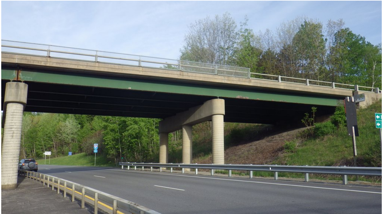
Figure 3.3: Facing I-91 Bridge 28 Southbound north abutment; note limited overhead clearance for drilling operations under existing bridge deck. [Inspection photo dated 2016]
