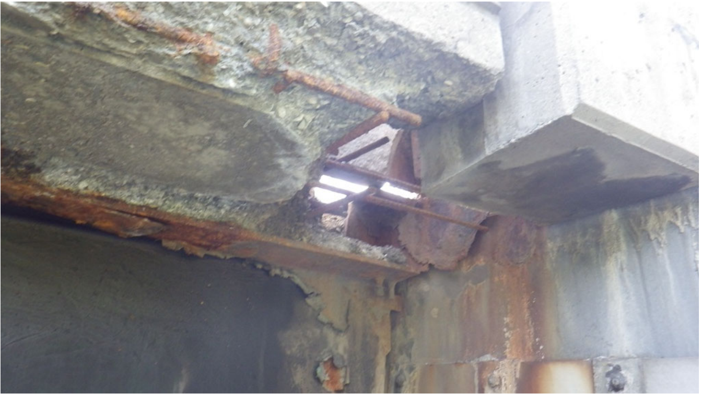
Deterioration at fascia and joint
