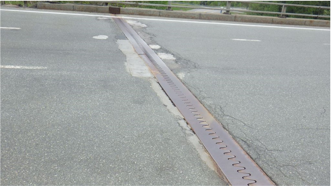
Deterioration around bridge joints
