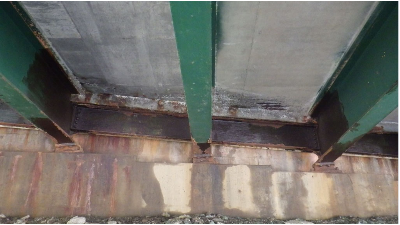
Abutment Condition (Note saturation due to leaky joint)
