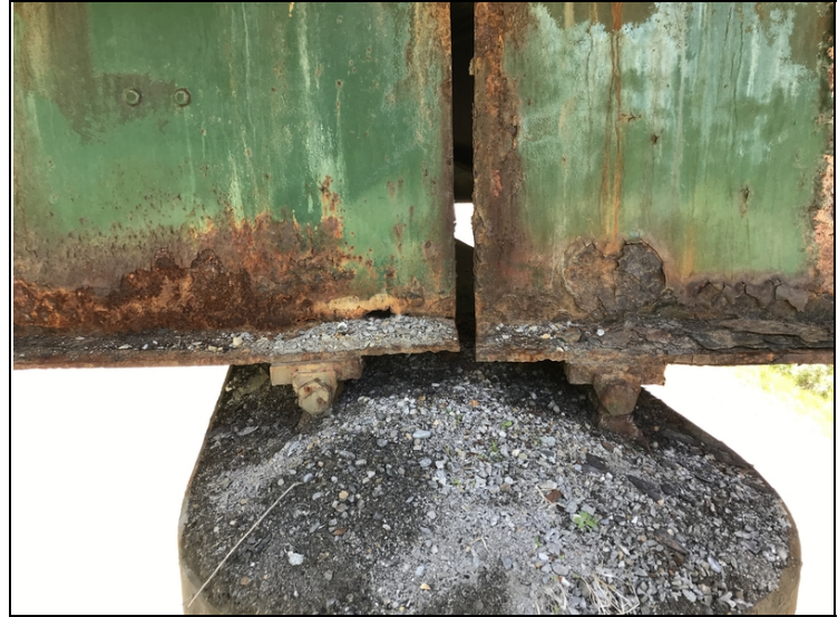
Span #2 Beams #1 Section Loss
