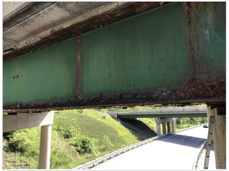
Beam #1 in Span #2 with Heavy Rust Scaling
