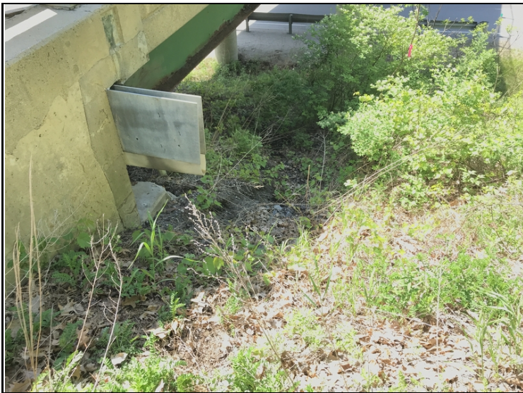
Erosion along Northwest Embankment
