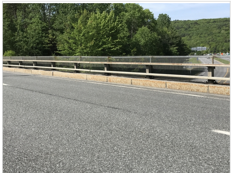
Sheared Connections Bolts along Snow Fence on West Side
