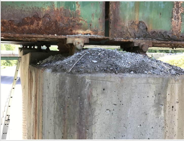
Heavy Debris on Pier #2 West End
