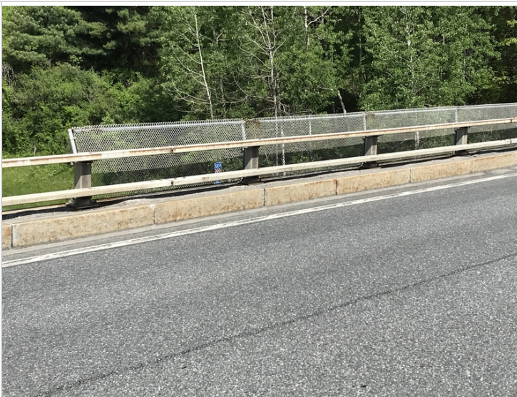
Western Snow Fence with Rusted Brackets and Frame
