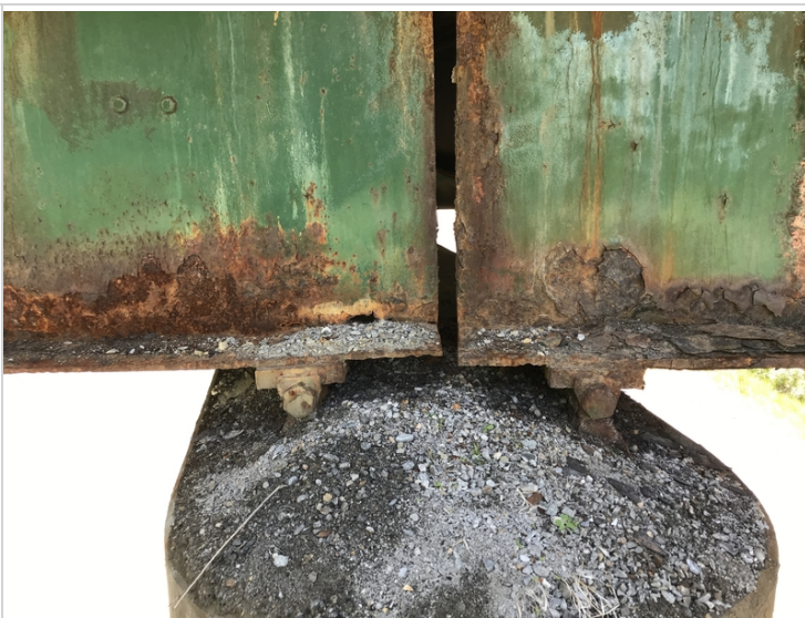
Span #2 Beams #1 Section Loss
