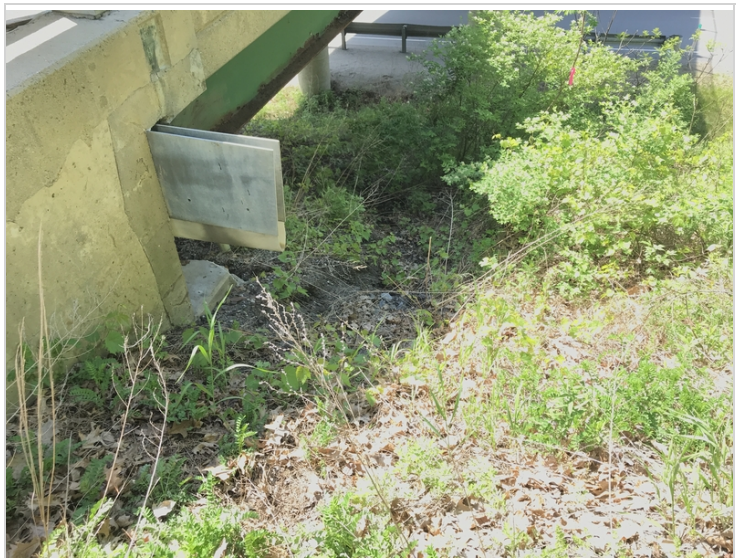
Erosion along Northwest Embankment
