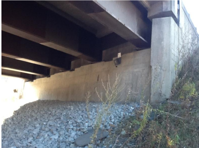
Camera on western bridge abutment
